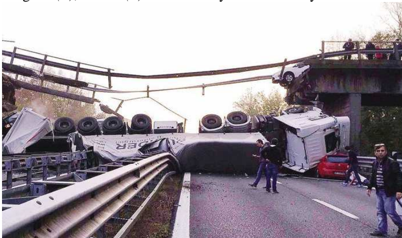
Figure 1 Collapse of Annone bridge in Italy under a 108 t truck in October 2016 (legal limit: 44 t)
