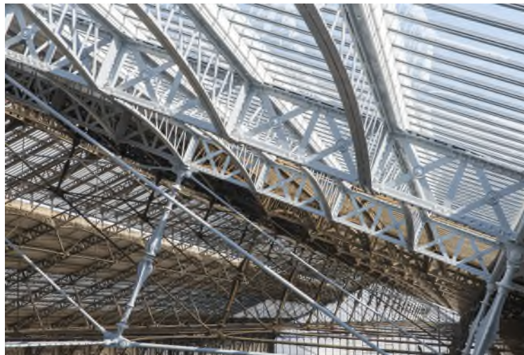
Figure 1: View of the roof structure of the railway station Gare d'Austerlitz built in 1869, under renovation in 2016, Paris, France (Picture from SNCF-AREP by M. Lee Vigneau).
