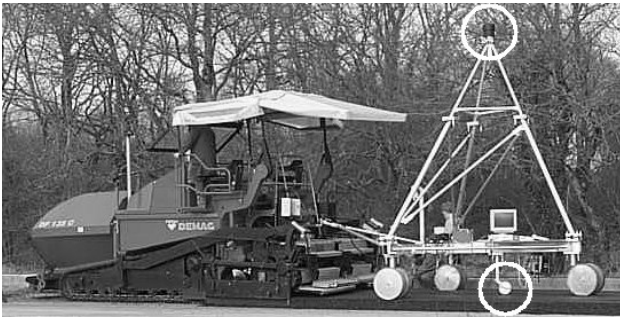
Figure 1: A CIRPAV demonstration: the LASERGUIDE is mounted on a trolley drawn by the asphalt paver and equipped with an encoder wheel
