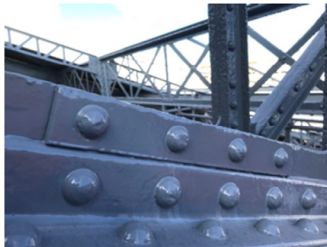
Figure 23: Local repair of a chord with added riveted plates in the train shed of Troyes renovated in 2021, Troyes, France (Picture from SNCF).
