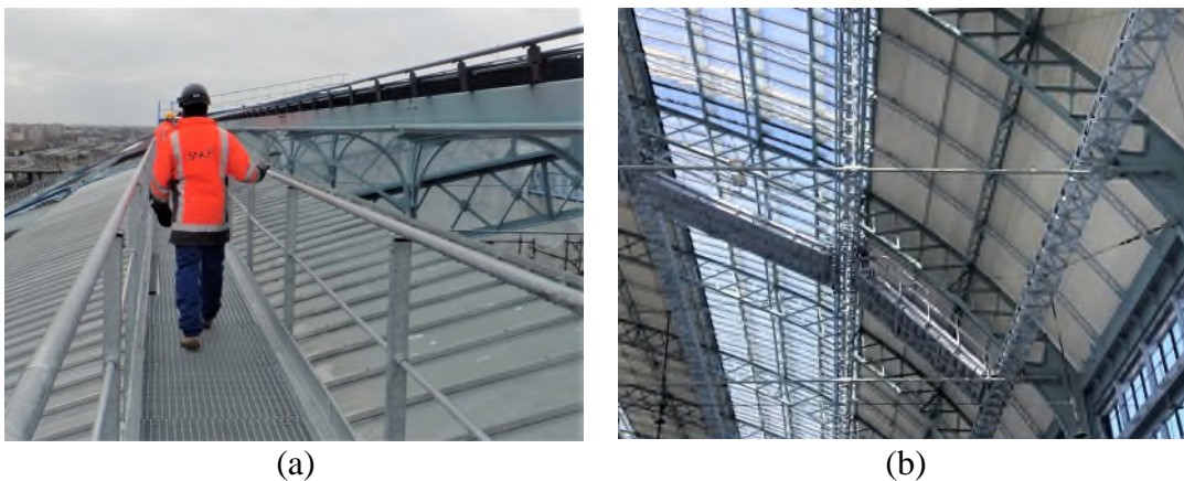
Figure 22 : Maintenance equipment added on the course of restoration projects in the train shed of Bordeaux Saint-Jean, Bordeaux, France (Pictures from SNCF and by H. Franz). (a) Maintenance platform and lifeline system over the roof, added in 2016 (picture: SNCF); (b) Metallic stairs and rails below the roof, added in 1928.
