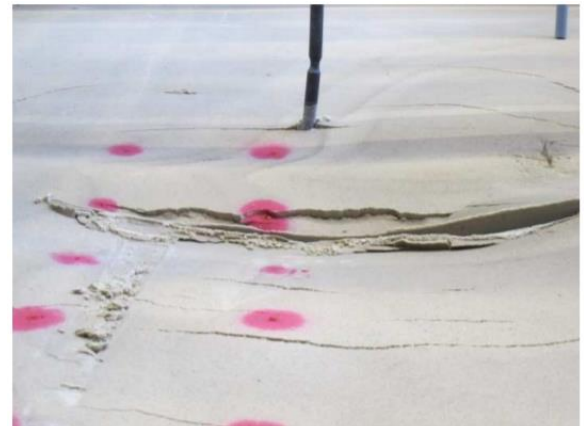
4. The soil deformation and pipe displacement before the sheet pile wall vibrates (initial situation), after the sheet pile wall has been vibrated in (sheet pile at deepest point) and after the sheet pile wall has been pulled out again was measured
