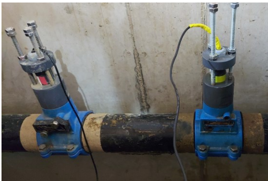
Fig. 2. Sensor installation in the Sense-city pipe
