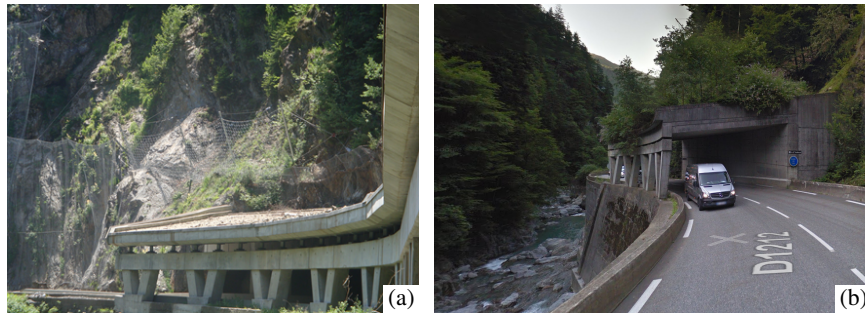
Fig. 1. Example of a rock shed gallery in Val d'Arly (Ugine, French Alps).
