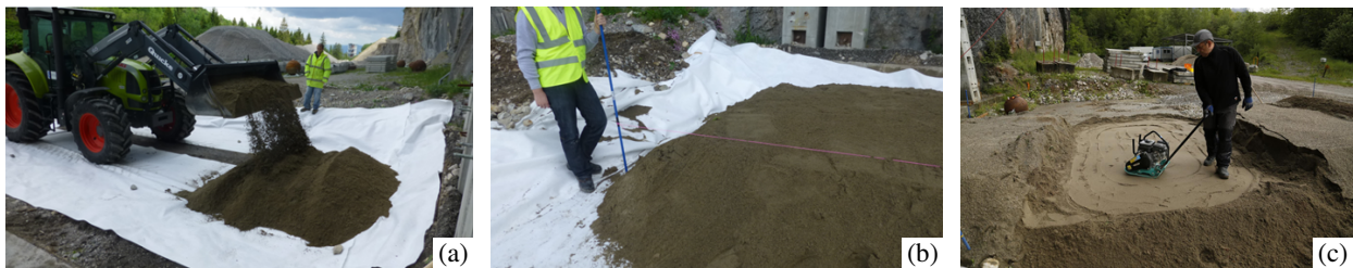
Fig. 4. (a) Soil dumping on geotextile using a backhoe; (b) Leveling of the soil sub-layers and (c) soil compaction using a vibrating plate compactor.
