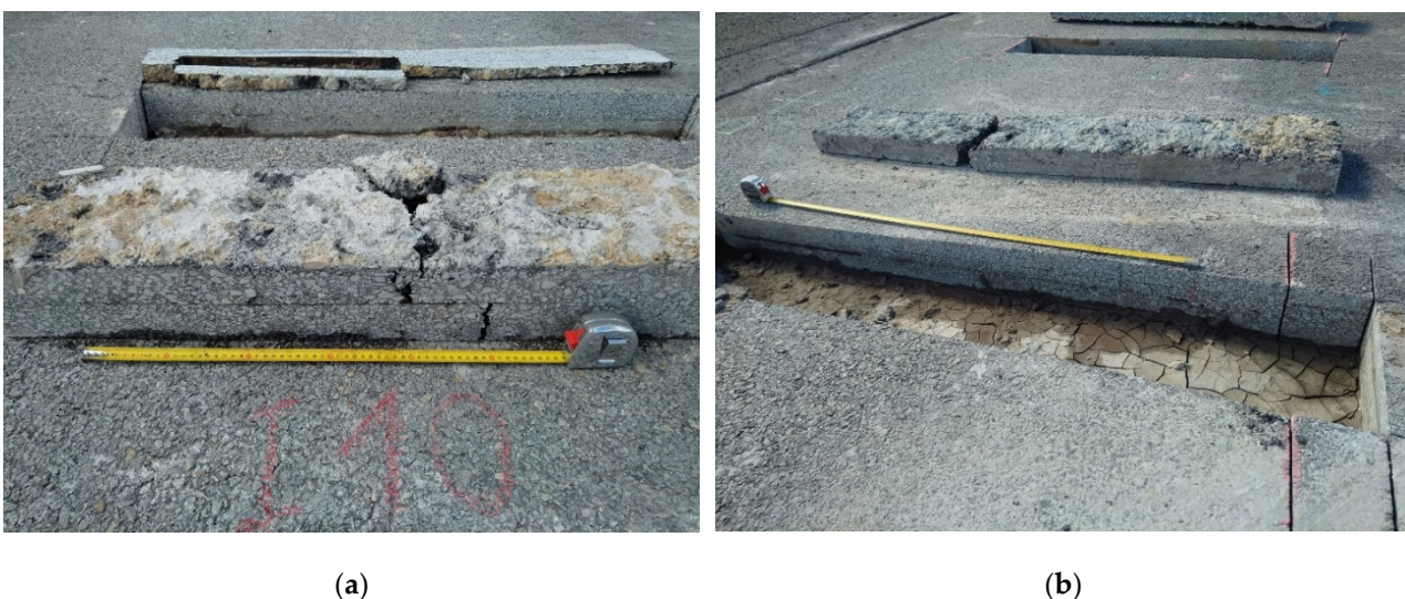
Figure 39. Transverse trenches and corresponding asphalt slabs of (a) defect I-10 and (b) defects I-12.
