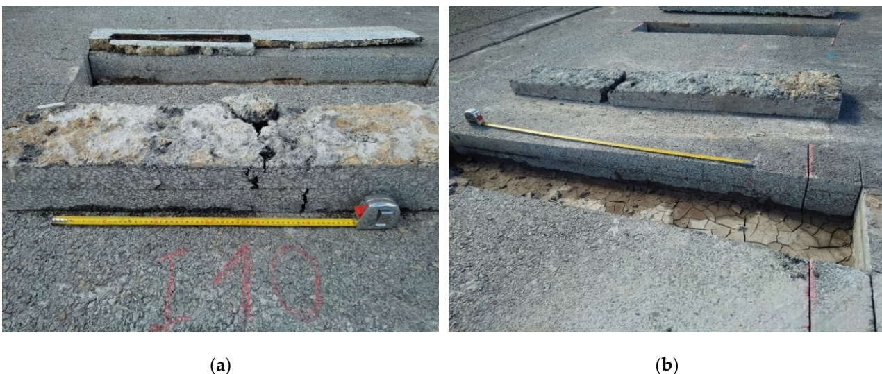
Figure 39. Transverse trenches and corresponding asphalt slabs of (a) defect I-10 and (b) defects I-12.
