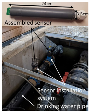
Fig. 1. Two sensor nodes installed into a drinking water pipe and connected via USB cable to control computers.
